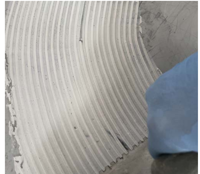
3 Wrong spreading leaving empty holes
