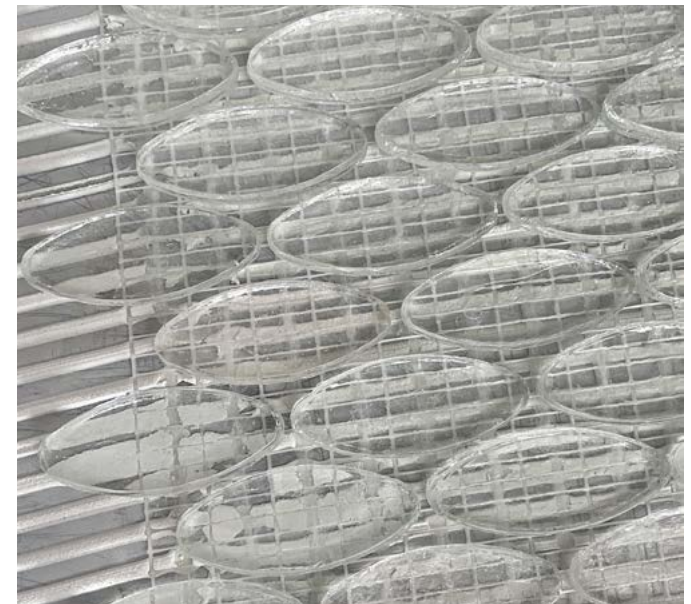
6 Visible empty holes under the clear glass mosaic and visible white fiber mesh
